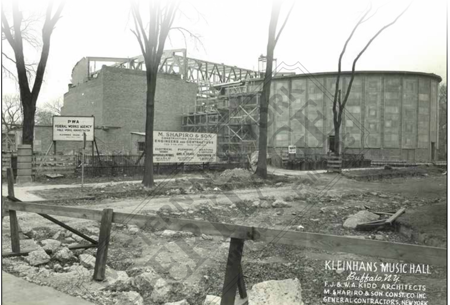
The familiar shape of Kleinmans Music Hall becomes apparent in this construction photo, ca. 1939. Visit wnyheritage.org for more engaging images of the hall being built. Kleinmans Music Hall
